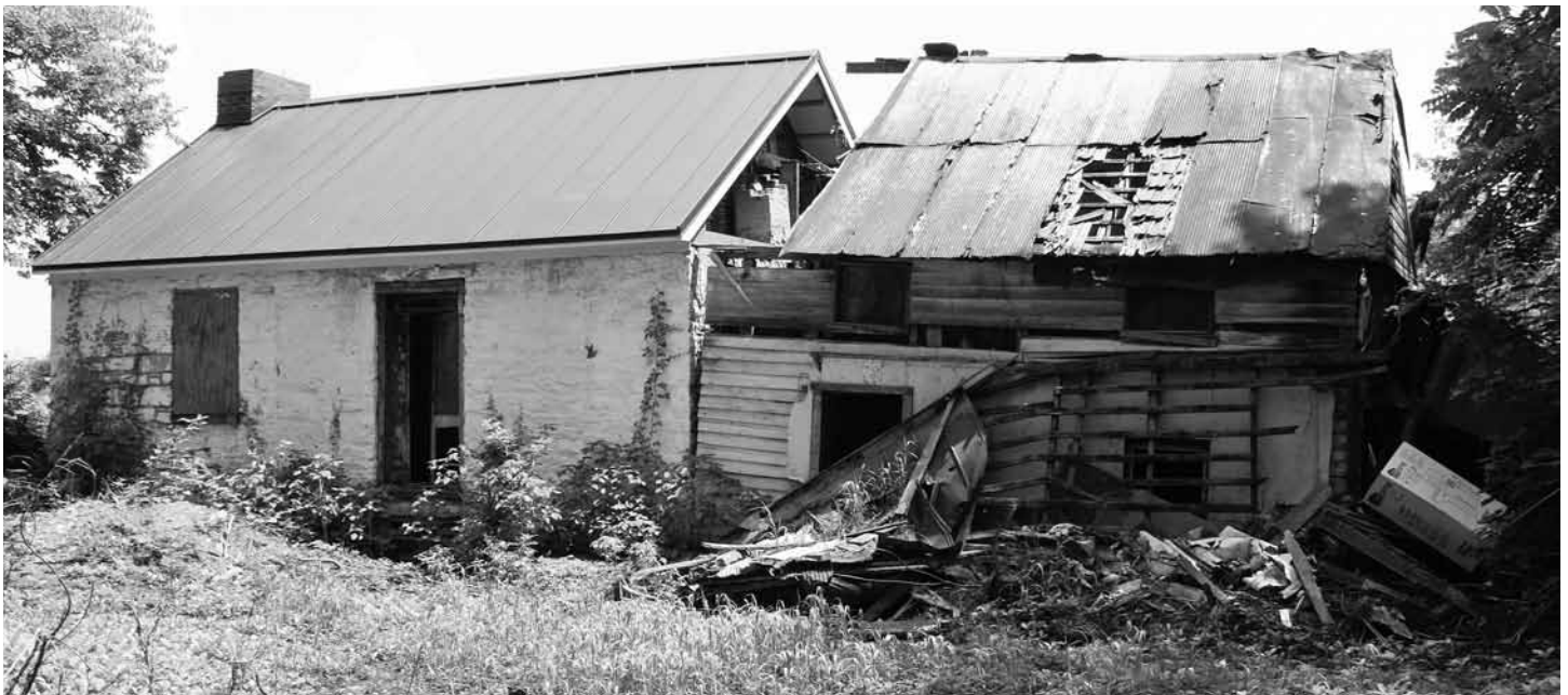
Duffields Station is open to some inspection on its north (back) side, where volunteers went in in 2008 to put a new tin roof on the stone segment of the building. The wooden section is probably beyond repair.
