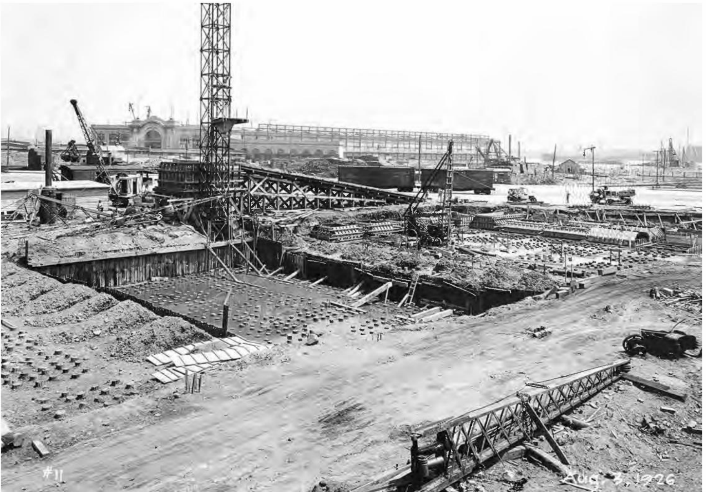
Construction of the Terminal, looking east toward the Delaware River, August 3, 1926. A Pere Marquette automobile and furniture car and a Lehigh Valley box car are on Delaware Avenue. The B&O foreign freight terminal at Pier 78 is in the background. (B&ORHS Archives)
