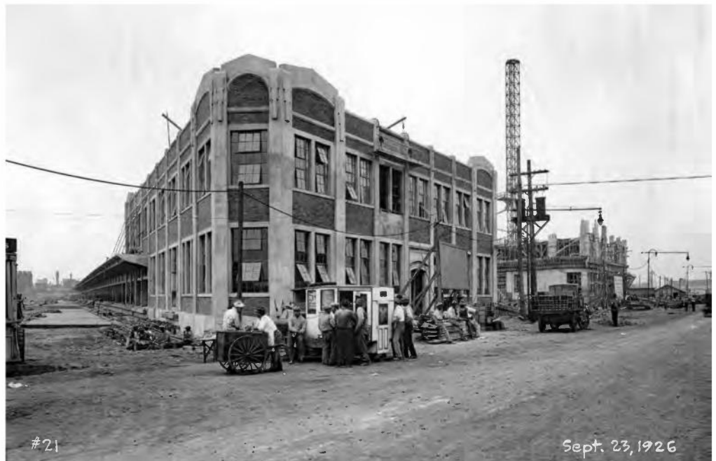
Construction of the Auction Sales Building and the Cold Storage Warehouse, September 23, 1926. The buildings use concrete curtain wall and brick construction. Fish cakes are just 5 cents at the lunch wagon. (B&ORHS Archives)
