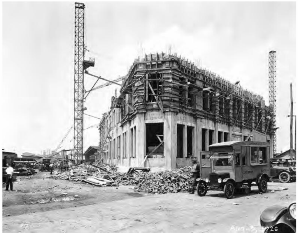
Construction of the Auction Sales Building, looking west from Delaware Avenue, August 3, 1926. The lunch wagon is advertising lemonade, root beer, ice cream, and hot dogs. (B&ORHS Archives)
