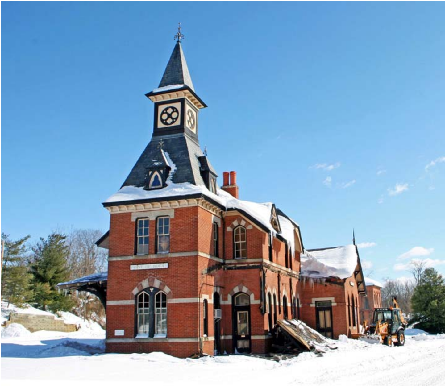
View of the Point of Rocks station looking east, showing the fallen platform cover.
