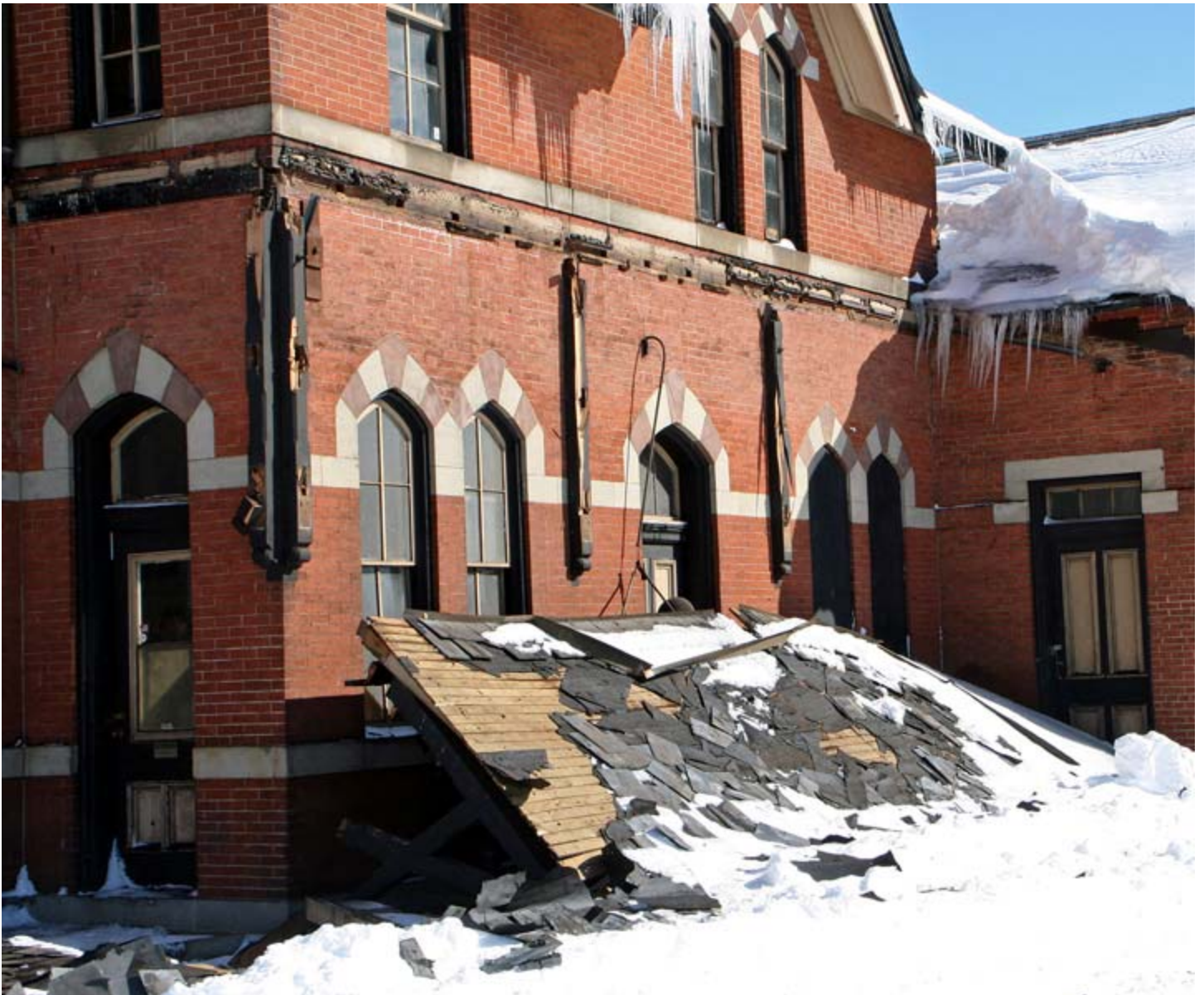
The old wooden cover over the platform adjacent to track 1 had fallen onto the platform from the weight of three feet of snow. This is on the south side of the station.
