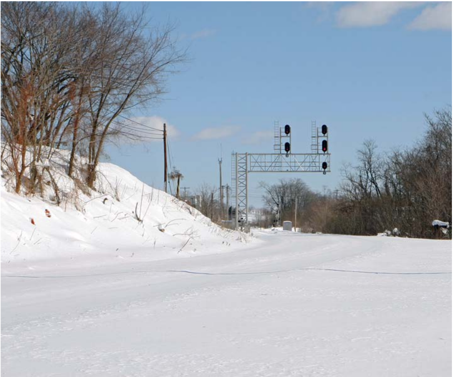
View of the Old Main Line looking to the east. The connection to the Metropolitan Sub, which MARC trains to Frederick use, is on the right. None of the tracks had been plowed.
